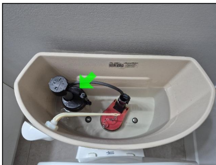
12. Flush mechanism inoperative
