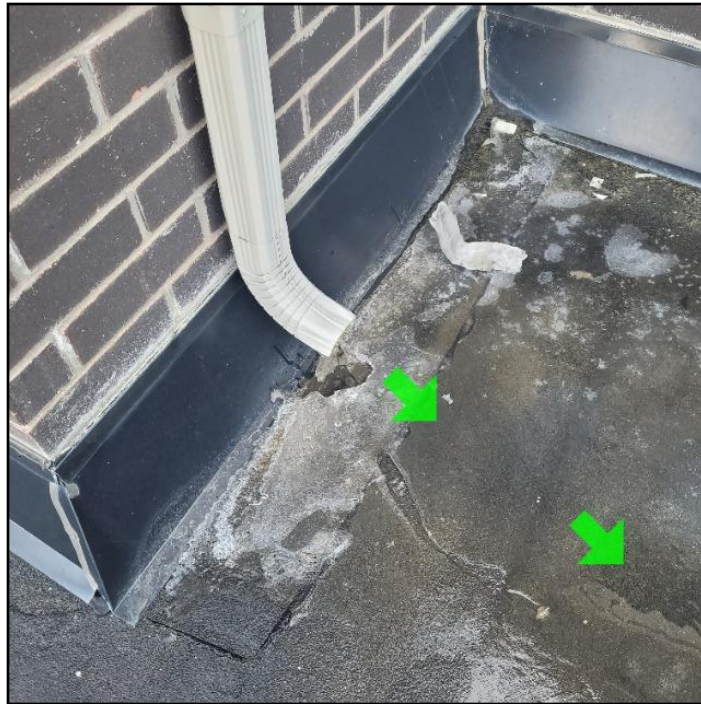
4. Discharge too close to building
